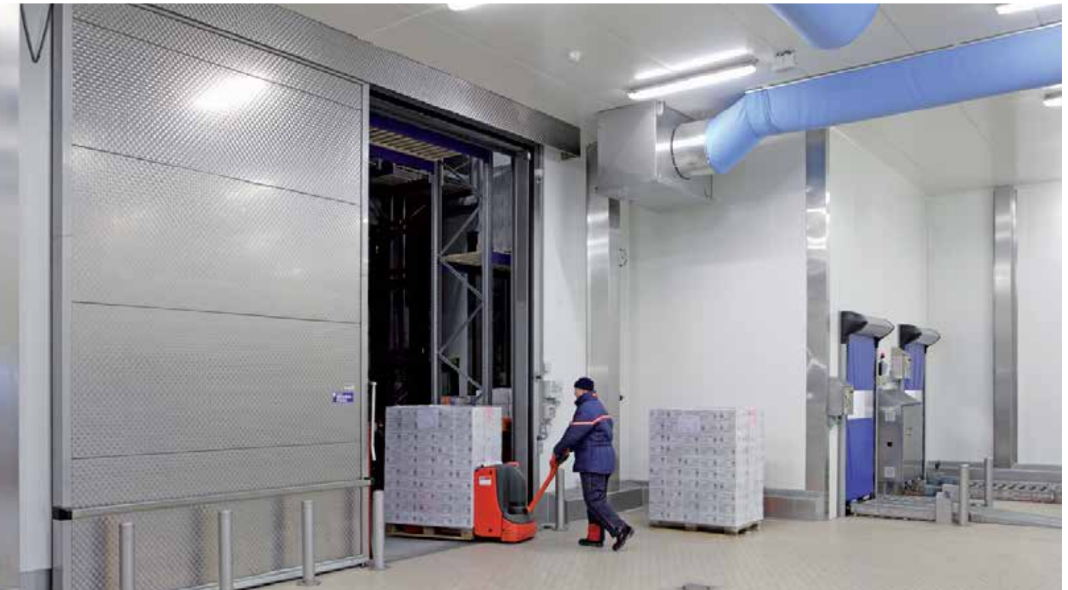
STAINLESS STEEL DOORS (CHILLER & FREEZER)
