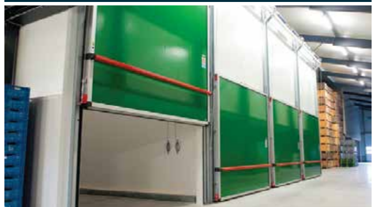
CONTROLLED ATMOSPHERE (CA) DOORS
