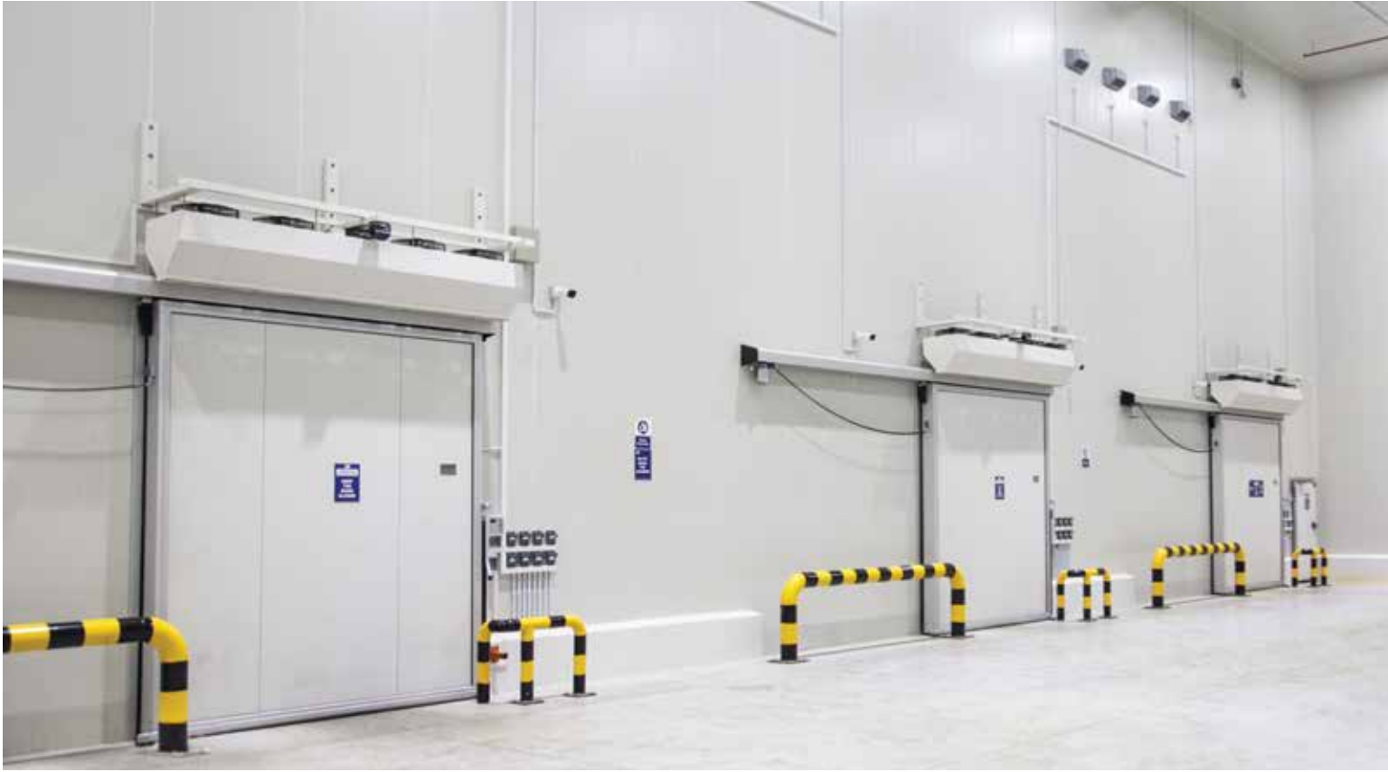
COLD STORE SLIDING DOORS (CHILLER & FREEZER)
